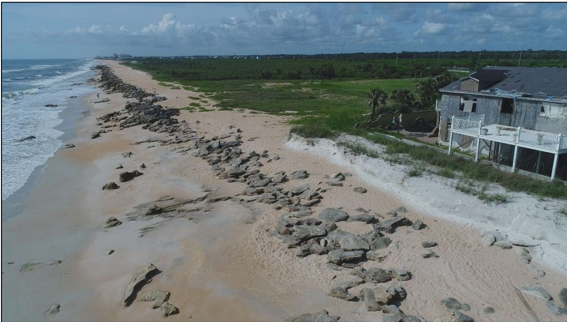
Figure 4.3: Typical conditions beach and dune conditions along Area 2 (09 November 2021); Matanzas Shores.
