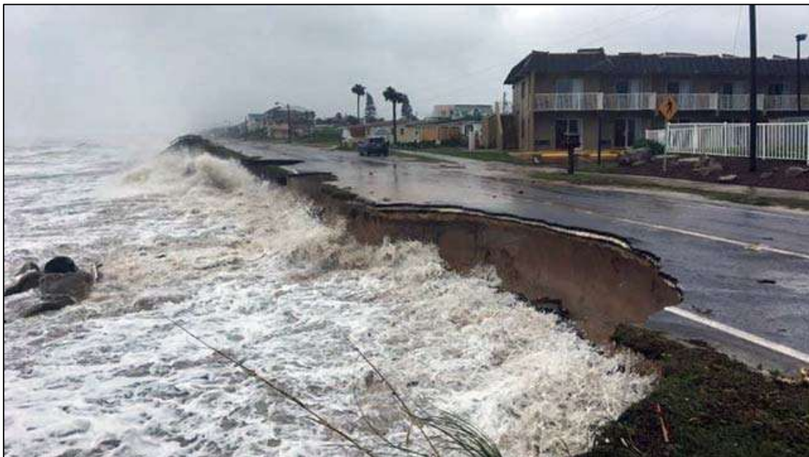
Figure 2.19: Example of complete beach and dune loss as well as impacts to SR A1A during Hurricane Matthew (October 2016) along the southern Flagler County Atlantic Ocean shoreline.
