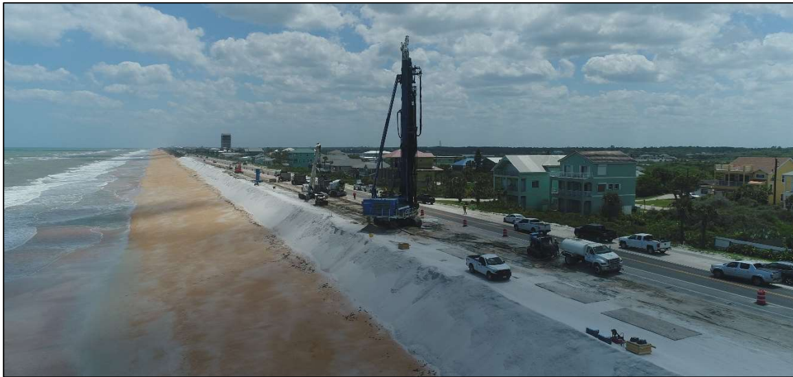
Figure 2.11: Construction of the FDOT secant wall and dune in northern Flagler Beach/southern Beverly Beach.
