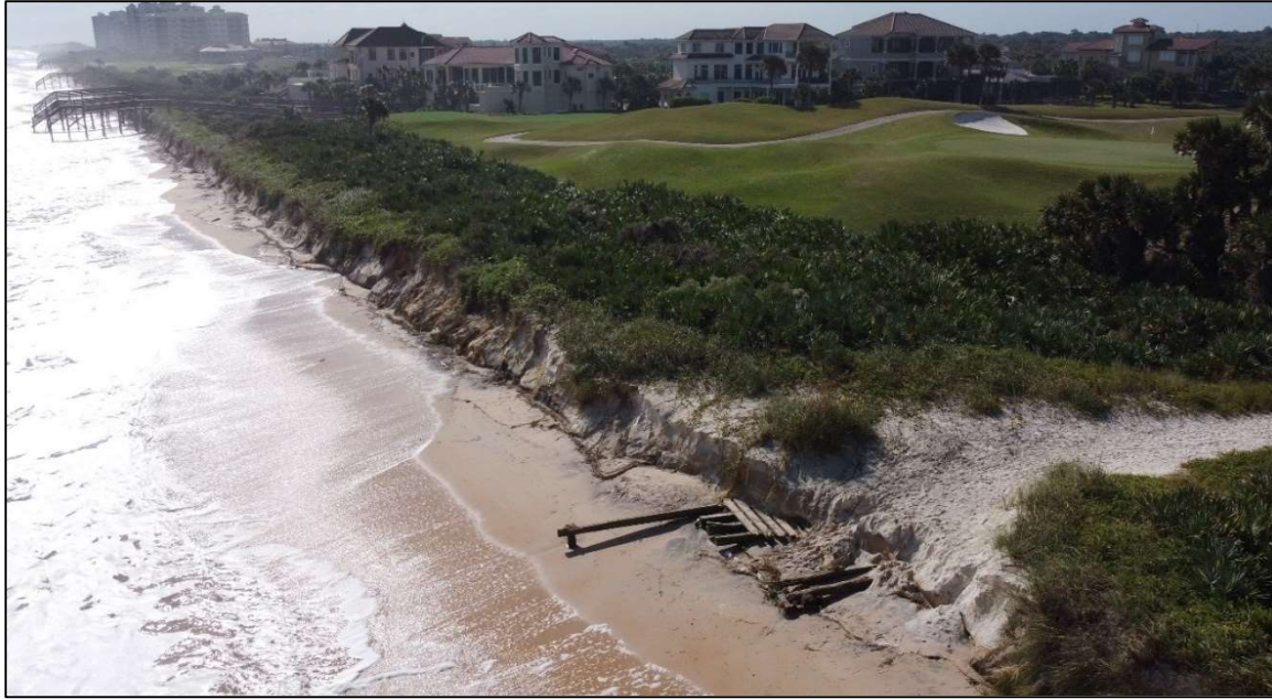
Figure 2.23: Damage from the November 2021 nor'easter at Jungle Hut Road Park and northern Hammock Dunes (R-35), 09 November 2021.
