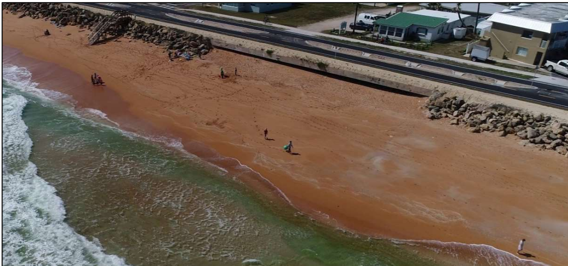
Figure 2.13: The 140-ft segment of seawall (R-82) that located within the larger rock revetment in the City of Flagler Beach (18 March 2020).
