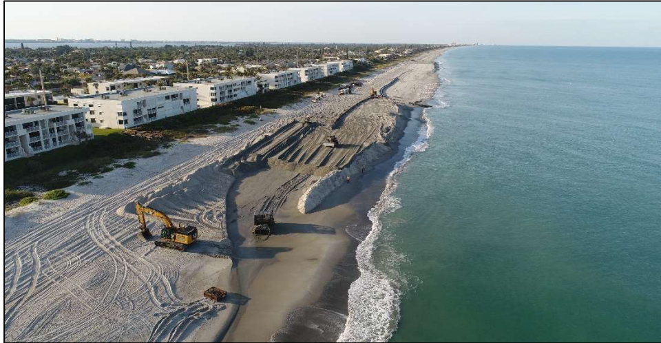
Figure 12.1: Construction of the stockpile in 2021 along the Mid-Reach in Brevard County, FL to avoid nearshore rock.
