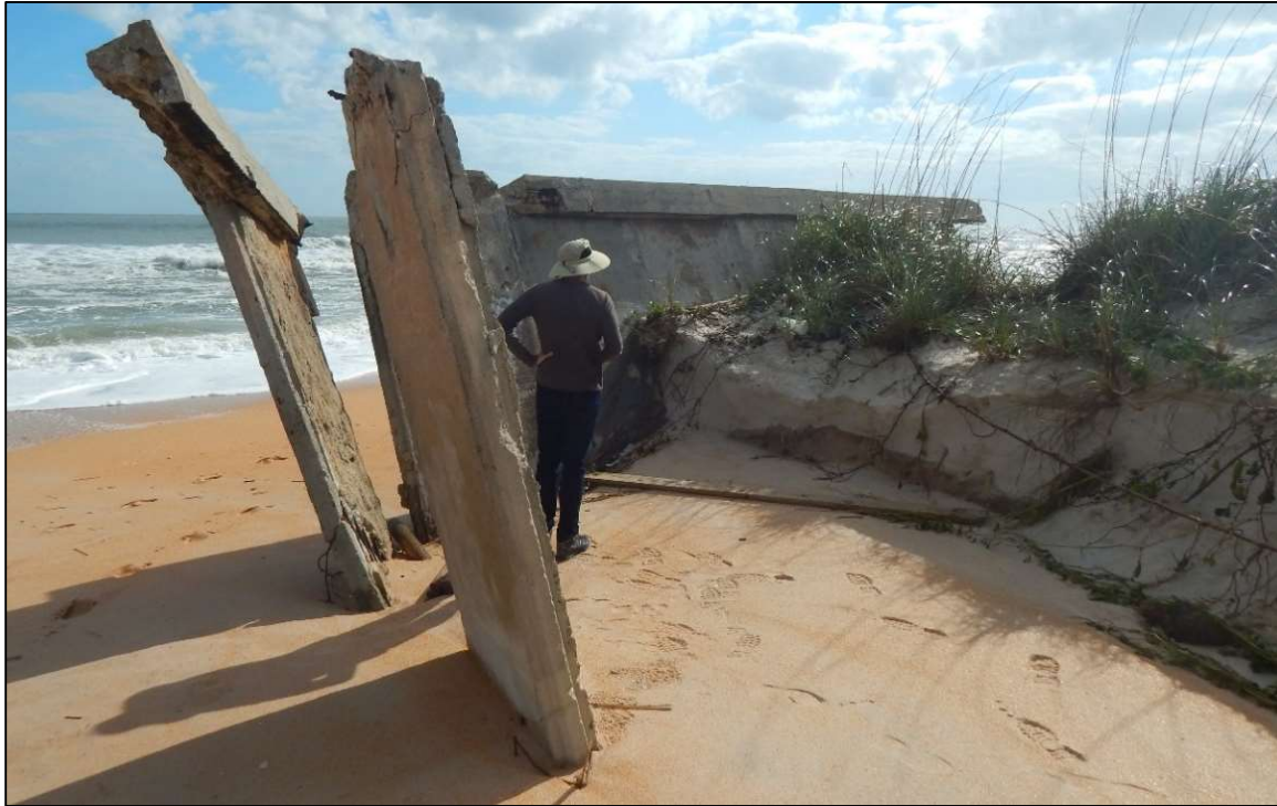
Figure 2.8: Remnants of the seawall at Varn Park, 9 November 2021.
